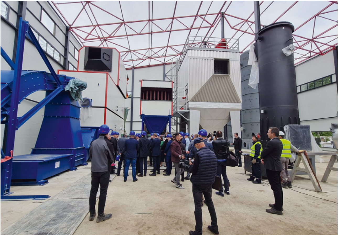
New biomass fuel plant in Priboj, which will contribute to the increase in use of renewable energy sources in Serbia to reduce pollution. Project 'Renewable Energy for District Heating Programme in Serbia'
