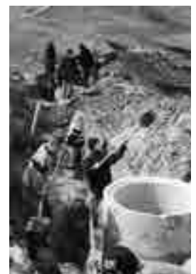
Local population contributing to the construction of a wastewater disposal line in Moldova.
